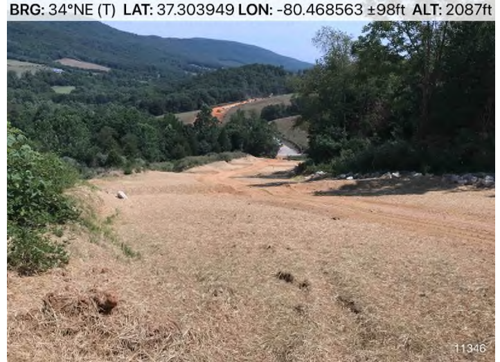
Figure 4: STA 11346+00 – Controls in place and functioning properly. BRG: 34°NE (T) LAT: 37.303949 LON: -80.468563 ±98ft ALT: 2087ft
