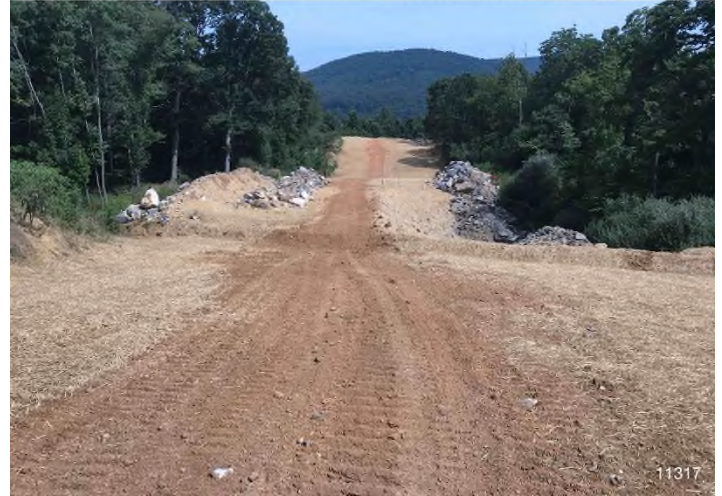
Figure 2: STA 11317+00 – Controls in place and functioning properly. BRG: 37°NE (T) LAT: 37.295694 LON: -80.476087 ±7237ft ALT: 2312ft
