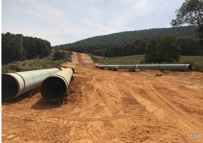
Figure 1: STA 11299+00 – Controls in place and functioning properly. BRG: 100°E (T) LAT: 37.296728 LON: -80.478602 ±32ft ALT: 2287ft
