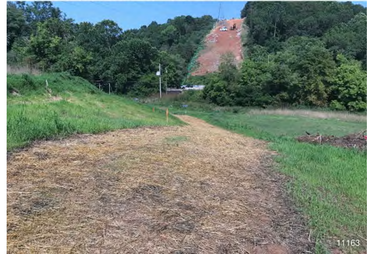
Figure 4: STA 11163+00 – Controls in place and functioning properly. BRG: 288°W (T) LAT: 37.311321 LON: -80.514494 ±16ft ALT: 1829ft
