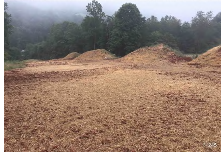
Figure 2: STA 11245+00 – Controls in place and functioning properly. BRG: 151°SE (T) LAT: 37.310473 LON: -80.506968 ±12326ft ALT: 2127ft
