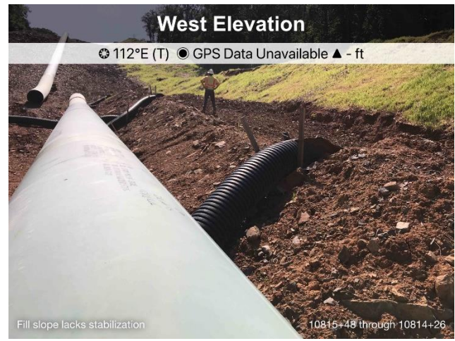
Figure 2: Two tone area lacks stabilization from 10815+45-10814+26
