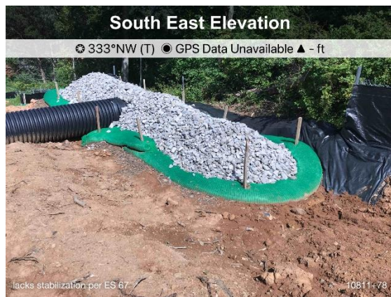
Figure 3: St10811+78 lacks stabilization per ES 67
