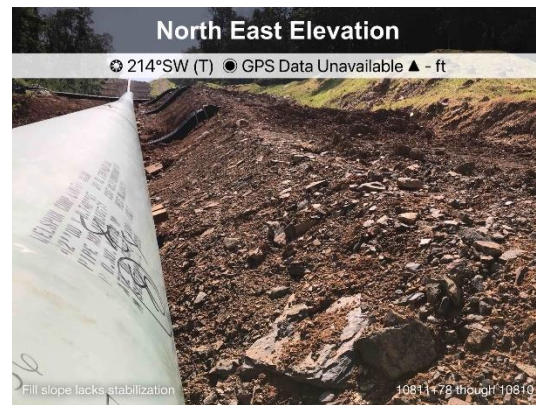
Figure 3: St10811+78 to10810 two tone area lacks stabilization
