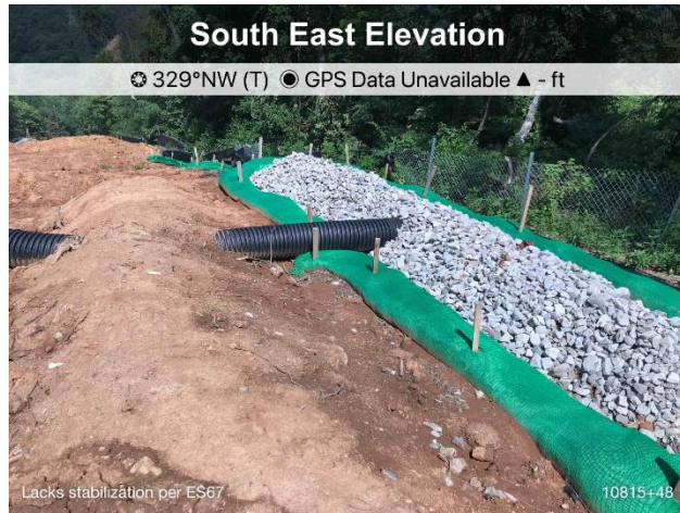
Figure 1: St10815+45 lacks stabilization per ES 67
