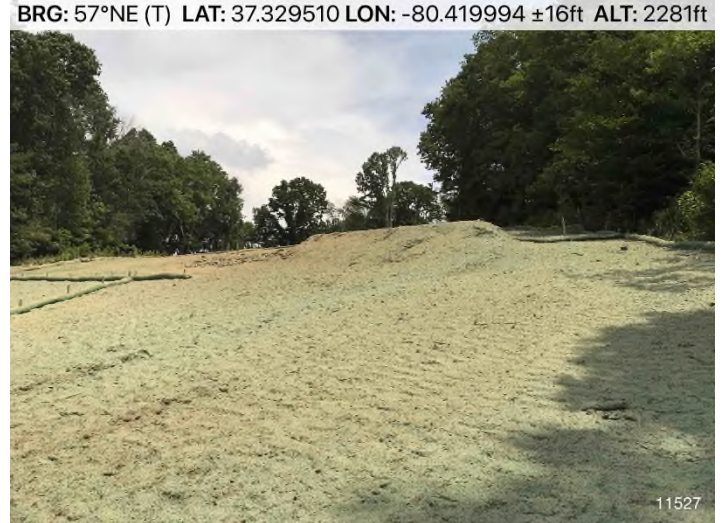
Figure 4: STA 11527+00 – Controls in place and functioning properly. BRG: 57°NE (T) LAT: 37.329510 LON: -80.419994 ±16ft ALT: 2281ft
