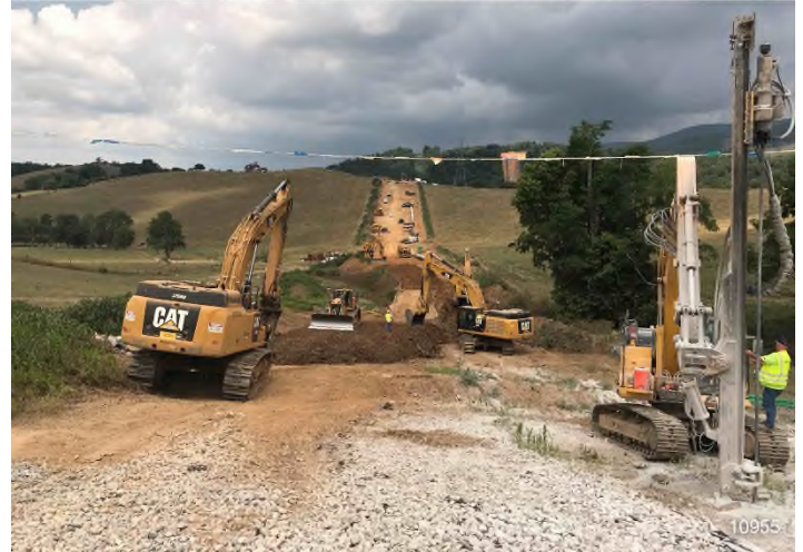
Figure 2: STA 10955+00 – Controls in place and functioning properly. BRG: 295°NW (T) LAT: 37.324559 LON: -80.588027 ±18789ft ALT: 2247ft
