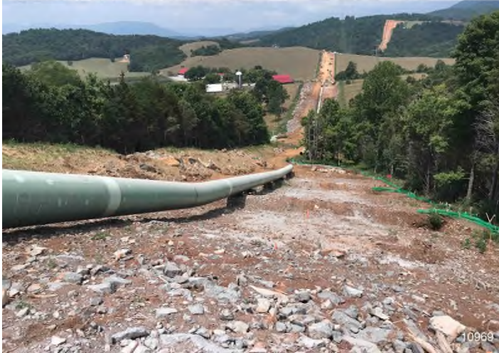
Figure 1: STA 10969+00 – Controls in place and functioning properly. BRG: 266°W (T) LAT: 37.327408 LON: -80.569155 ±164ft ALT: 2452ft
