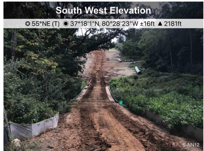
Figure 2: Designated crossing S-NN12
