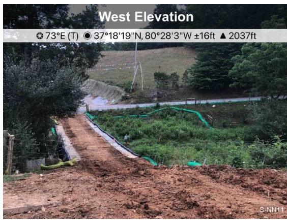
Figure 3: Designated crossing S-NN11
