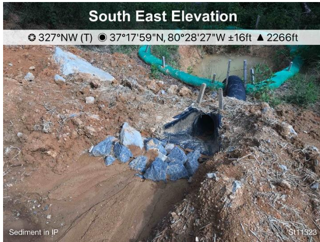
Figure 1: St11323 inlet protection requires sediment removal
