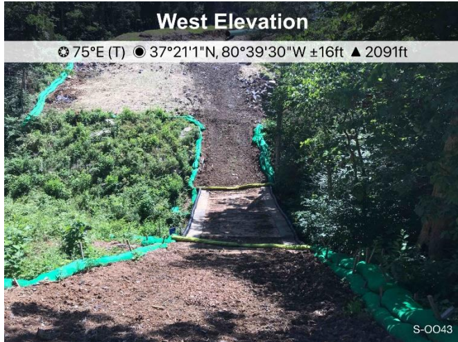
Figure 5: Designated crossing S-0043, ECD's are in place.
