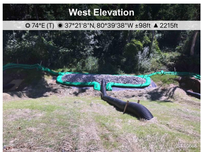
Figure 8: ECD has been installed at St10669
