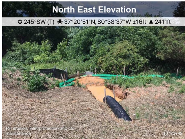
Figure 5: St 10725+42 CFS requires sediment removal
