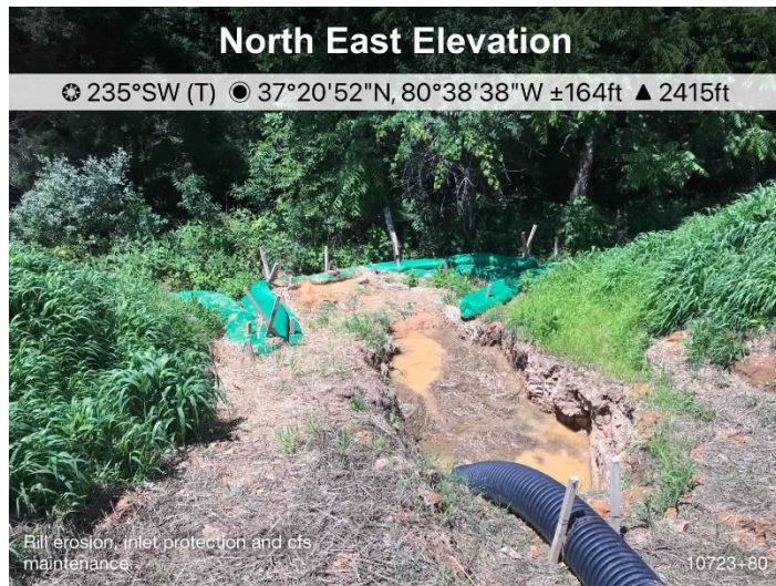
Figure 3: St10723+80 CFS requires sediment removal
