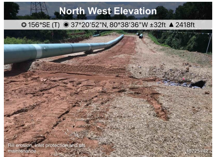
Figure 4: St 10725+42 rill erosion and sediment in inlet protection
