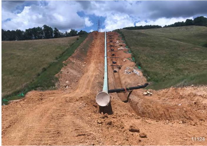
Figure 3: STA 11124+00 – Controls in place and functioning properly. BRG: 279°W (T) LAT: 37.315474 LON: -80.526587 ±16ft ALT: 1946ft
