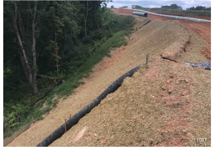
Figure 4: STA 11087+00 – Controls in place and functioning properly. BRG: 263°W (T) LAT: 37.315434 LON: -80.538351 ±16ft ALT: 2171ft
