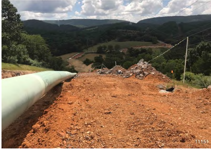
Figure 1: STA 11151+00 – Controls in place and functioning properly. BRG: 103°E (T) LAT: 37.312516 LON: -80.518535 ±16ft ALT: 2029ft
