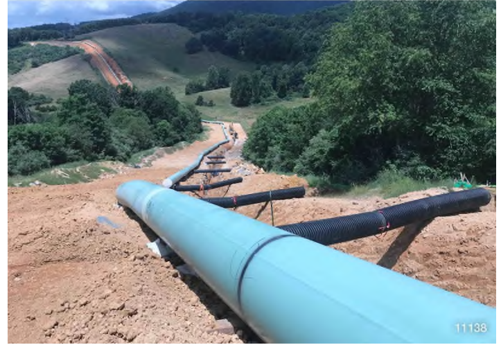
Figure 2: STA 11138+00 – Controls in place and functioning properly. BRG: 285°W (T) LAT: 37.312907 LON: -80.518180 ±15492ft ALT: 2143ft
