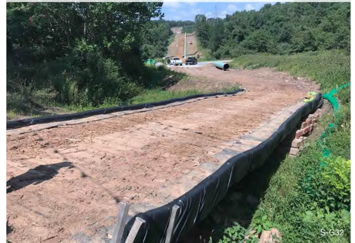
Figure 4: Stream S-G32 – Controls in place and functioning properly. BRG: 298°NW (T) LAT: 37.344473 LON: -80.663359 ±7417ft ALT: 2129ft
