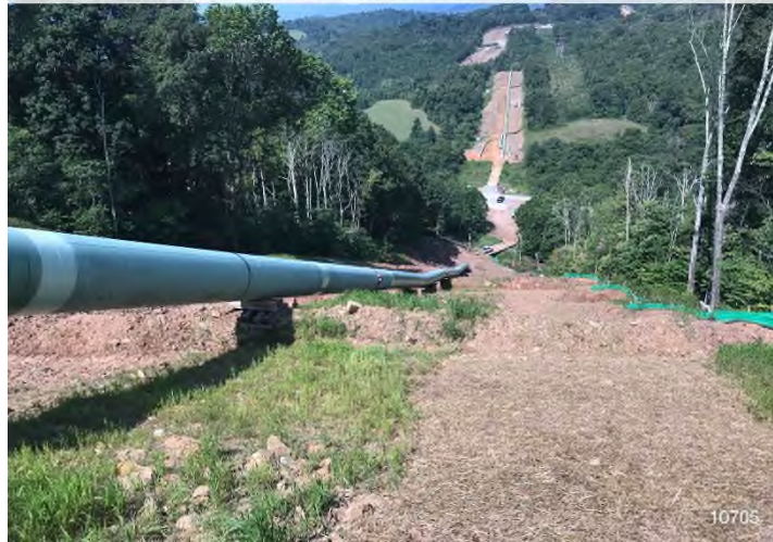
Figure 3: STA 10705+00 – Controls in place and functioning properly. BRG: 270°W (T) LAT: 37.339618 LON: -80.660111 ±19573ft ALT: 2332ft
