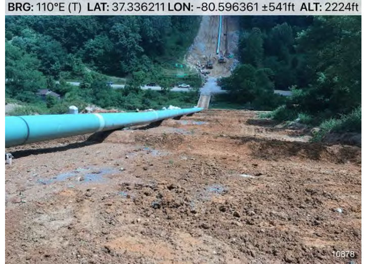
Figure 4: STA 10878+00 – Controls in place and functioning properly. BRG: 110°E (T) LAT: 37.336211 LON: -80.596361 ±541ft ALT: 2224ft
