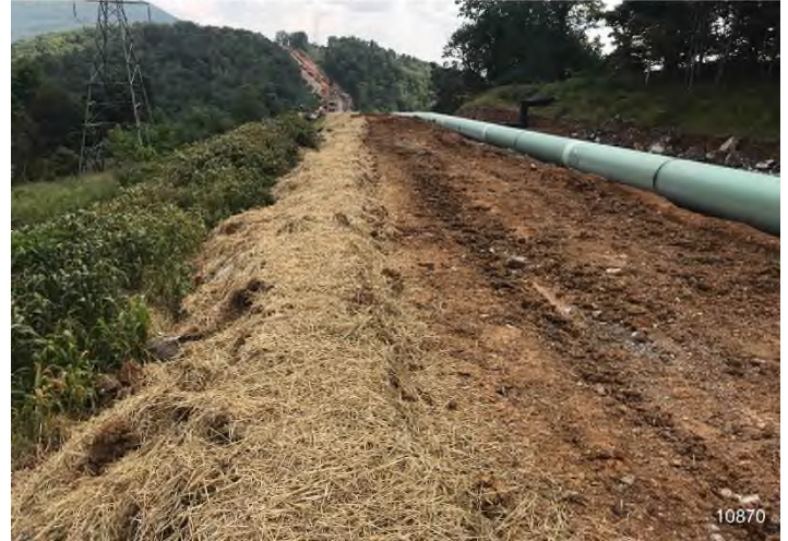
Figure 2: STA 10870+00 – Controls in place and functioning properly. BRG: 114°SE (T) LAT: 37.336352 LON: -80.601044 ±32ft ALT: 2448ft
