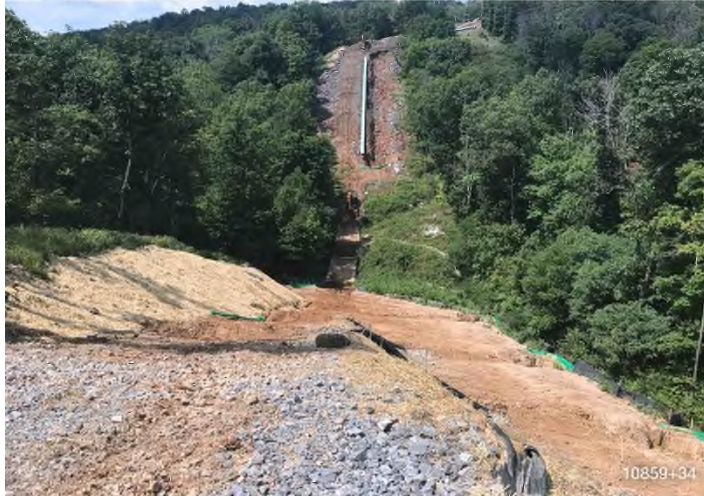
Figure 1: STA 10859+34 – Controls in place and functioning properly. BRG: 310°NW (T) LAT: 37.337414 LON: -80.604308 ±16ft ALT: 2326ft
