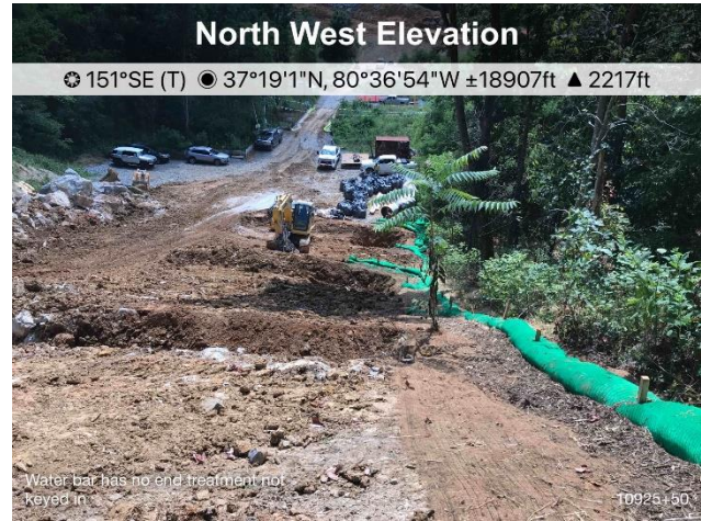
▪ Figure 6: St 10925+50 water bar has no end treatment
