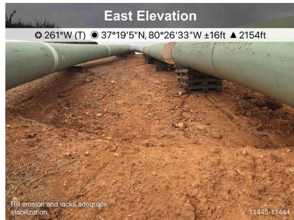
Figure 2: St 11444-11445 lacks stabilization and rill erosion has occurred.
