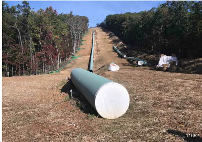
Figure 1: STA 11682+00 – Controls in place and functioning properly. Area stabilized with straw. BRG: 332°NW (T) LAT: 37.300374 LON: -80.392584 ±16ft ALT: 2576ft
