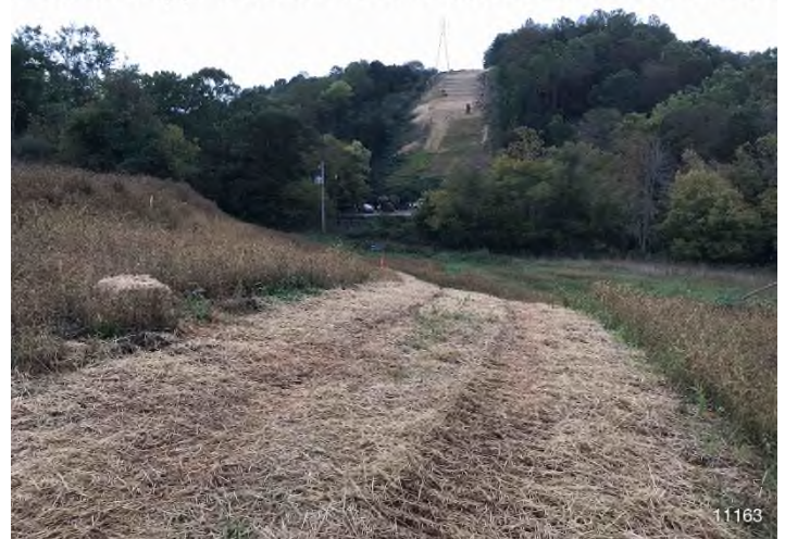
Figure 4: STA 11163+00 – Controls in place and functioning properly. BRG: 288°W (T) LAT: 37.311478 LON: -80.514426 ±98ft ALT: 1862ft
