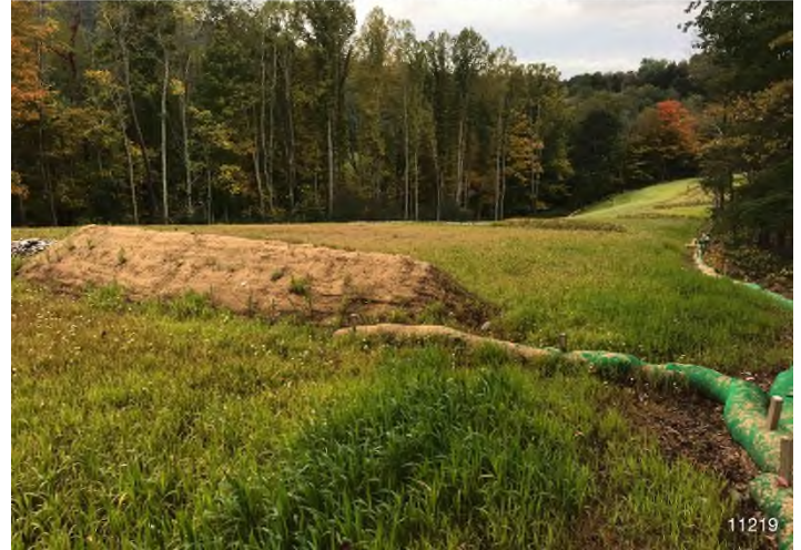
Figure 2: STA 11219+00 – Controls in place and functioning properly. BRG: 273°W (T) LAT: 37.301544 LON: -80.504047 ±16ft ALT: 2069ft
