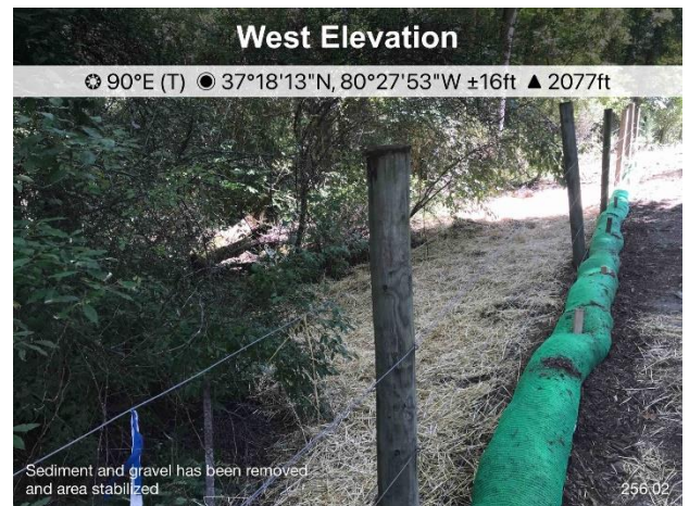
Figure 4: Escaped sediment and gravel has been removed and the area has been stabilized.
