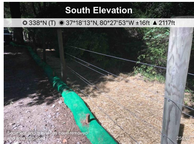
Figure 2: Escaped sediment and gravel has been removed and the area has been stabilized.
