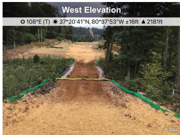
Figure 4: Designated crossing S-S4, ECD's are in place and functioning.
