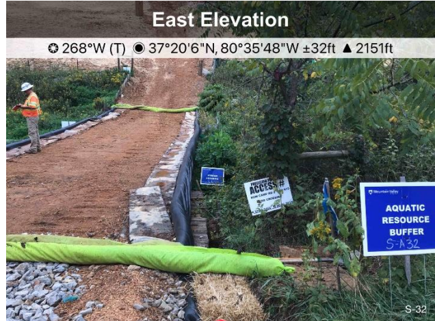
Figure 2: Designated crossing S-32, ECD's are in place and functioning.
