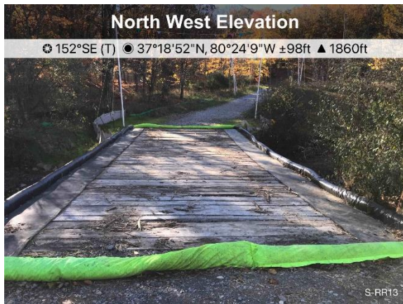
Figure 3: Designated crossing S-RR13, ECD's are in place.
