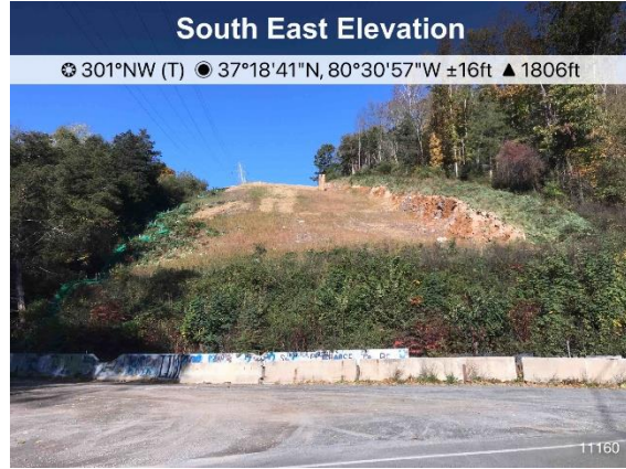
Figure 2: St 11160 Mountain Lake road crossing, ECD's are in place and slope is stabilized.
