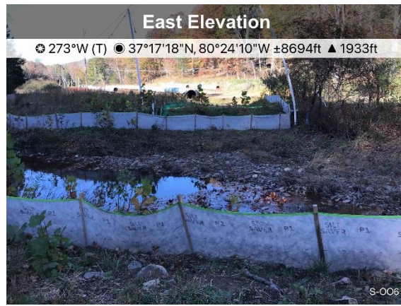
Figure 4: Designated crossing S-006, ECD's are in place.
