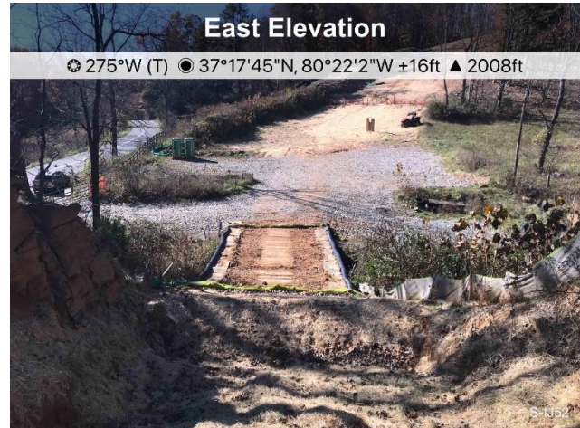
Figure 2: Designated crossing S-IJ52, ECD's are in place.
