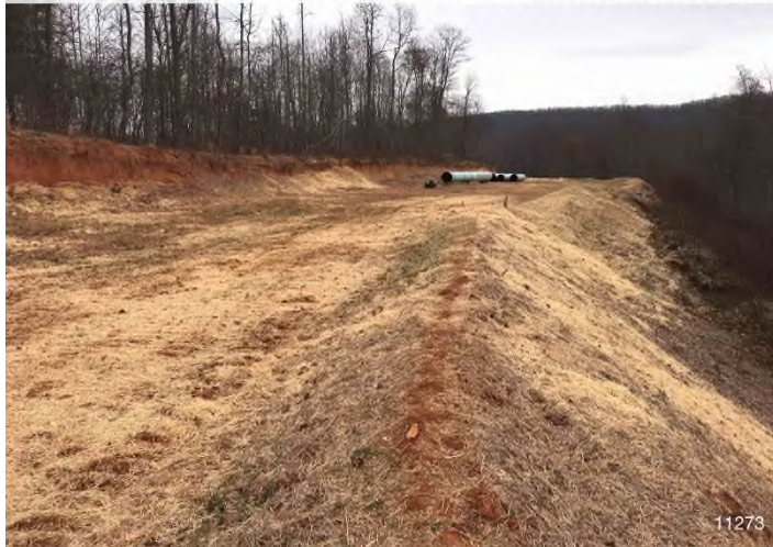
Figure 3: STA 11273+00 – Controls in place and functioning properly. Area stabilized with straw BRG: 84°E (T) LAT: 37.296367 LON: -80.488366 ±16ft ALT: 2285ft
