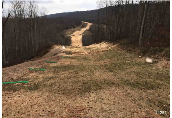
Figure 2: STA 11284+00 – Controls in place and functioning properly. Area stabilized with straw BRG: 72°E (T) LAT: 37.295938 LON: -80.484098 ±98ft ALT: 2120ft
