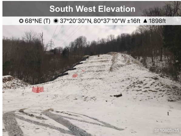
Figure 1: ESC controls were snow covered near St 10803+35
