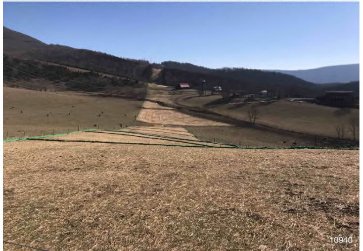
Figure 4: STA 10940+00 – Controls in place and functioning properly. Area stabilized with straw. BRG: 189°S (T) LAT: 37.330028 LON: -80.579988 ±16ft ALT: 2282ft
