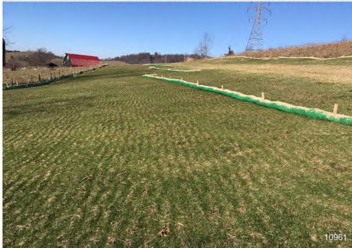
Figure 3: STA 10961+00 – Controls in place and functioning properly. BRG: 307°NW (T) LAT: 37.327940 LON: -80.572925 ±16ft ALT: 2308ft
