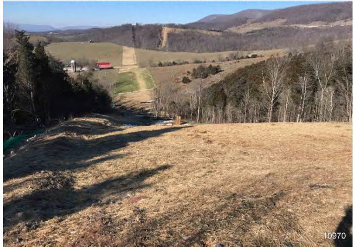
Figure 2: STA 10970+00 – Controls in place and functioning properly. Area stabilized with straw. BRG: 305°NW (T) LAT: 37.327106 LON: -80.570319 ±16ft ALT: 2452ft
