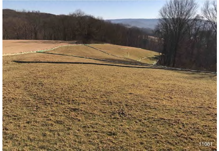
Figure 2: STA 11081+00 – Controls in place and functioning properly. BRG: 96°E (T) LAT: 37.316280 LON: -80.543244 ±13795ft ALT: 2238ft
