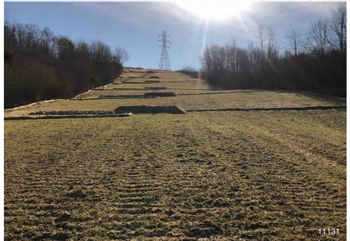
Figure 4: STA 11131+00 – Controls in place and functioning properly. BRG: 133°SE (T) LAT: 37.314253 LON: -80.523731 ±164ft ALT: 2050ft
