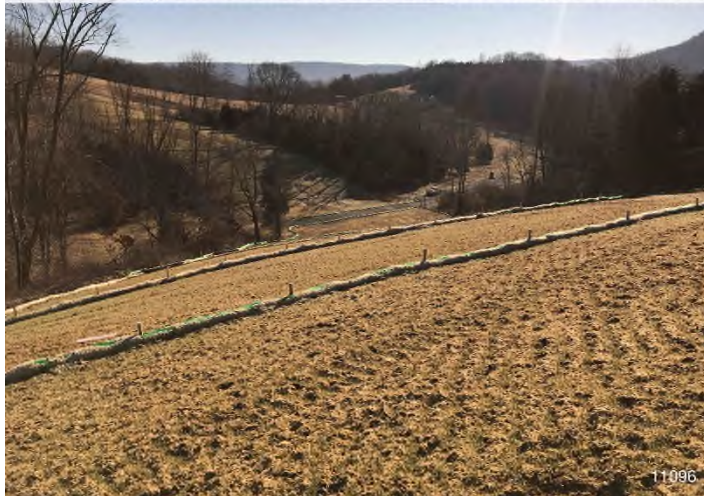
Figure 3: STA 11096+00 – Controls in place and functioning properly. BRG: 103°E (T) LAT: 37.313340 LON: -80.535043 ±98ft ALT: 1910ft
