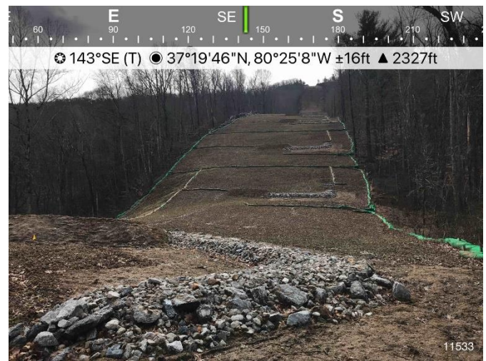
Figure 4: St1 1533, ECD's are in place and functioning.
