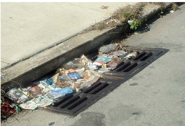
Figure 4.38. Trash Accumulated at a Curb Inlet. Source: Center for Watershed Protection
