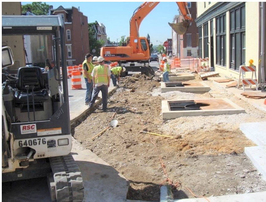
Figure 5-C.22. Construction of a Green Street in Baltimore, MD Source: Chesapeake Bay Stormwater Training Partnership
