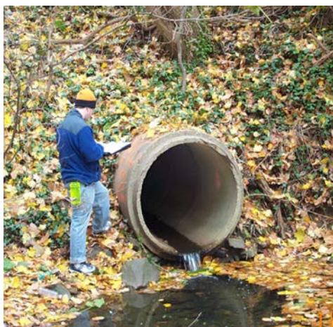
Figure 5-D.22. Suspicious Flow from Storm Drain Pipe Outlet
