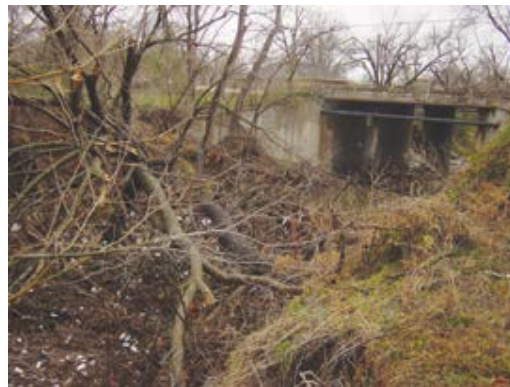
Figure 5-B.8. Fallen trees and debris resulting from stream erosion block a section of Imhoff Creek
