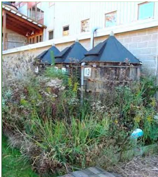
Figure 5-C.12. Rainwater Harvesting Cisterns
