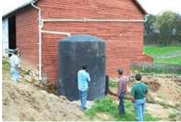
Figure 6-B.11. Cistern to Harvest Rainwater
