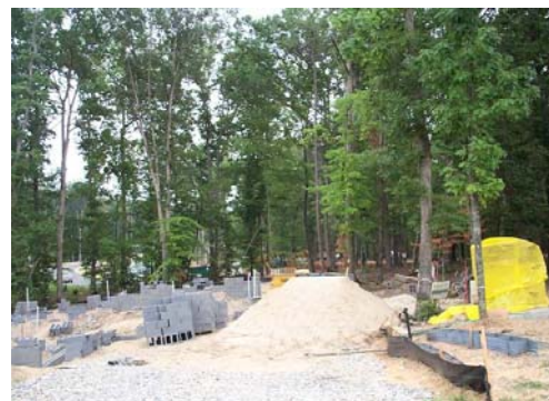
Figure 6.24. Construction Materials Stored Within Critical Root Zones of Trees Being Preserved Source: Center for Watershed Protection
