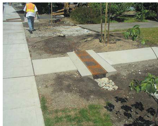
Figure 7.27. Designers need to find creative ways to pass runoff across driveways and sidewalks. Source: CWP, 2007a
