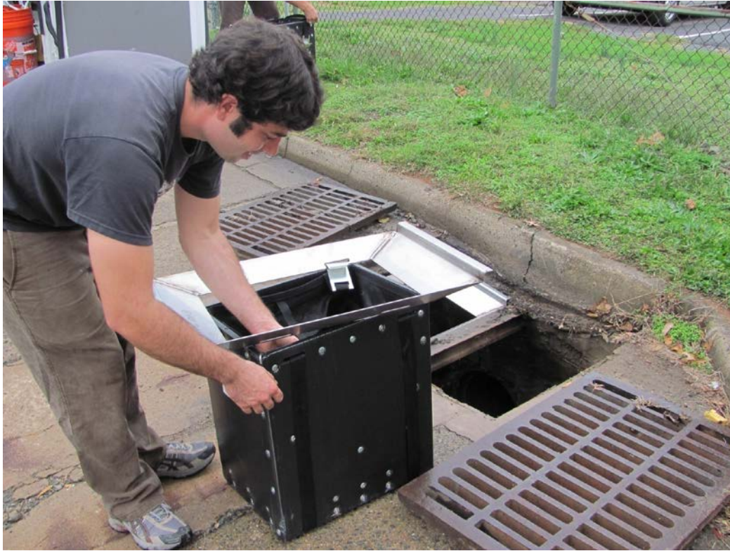
Figure 7-A.20. City Yard Catch Basin Filter Inserts
