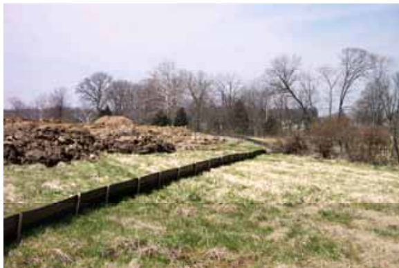
Figure 8.1. Temporary Silt Fence
