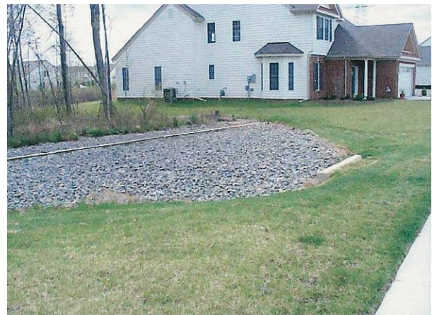
Figure 8.29. Filter Strip with Level Spreader (gravel pad as pre-treatment)
