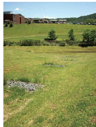
Good Conveyance: Good conveyance design can include check dams, Vegetation, and adequate channel lining.
