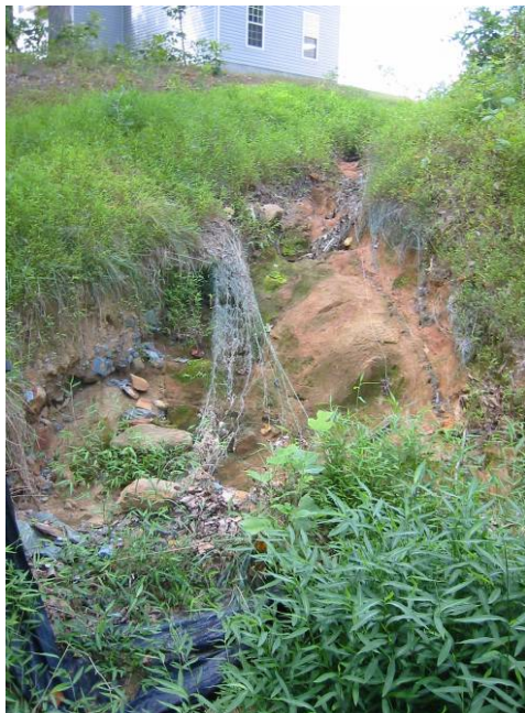
Figure 9.1. An unmaintained stormwater conveyance channel now generating sediment to the receiving channel (Source: CWP, 2009)
