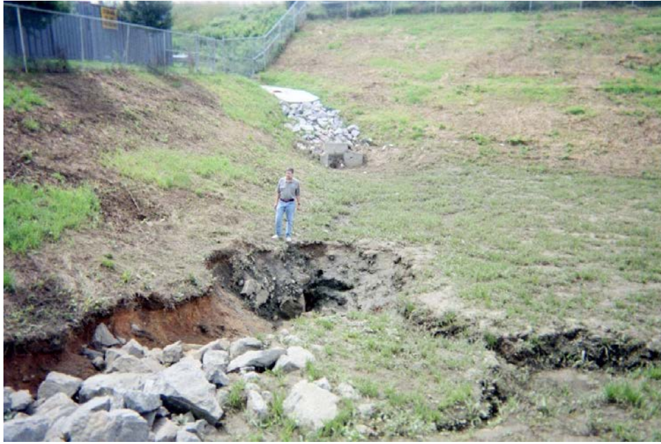
Figure 9.8. BMP Sinkhole Collapse
