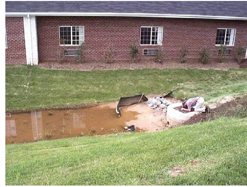
Bioretention area does not drain properly.
