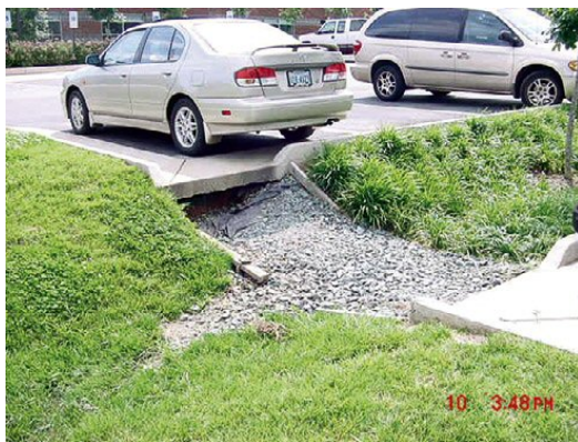
Curb inlets to bioretention swale have eroded.
