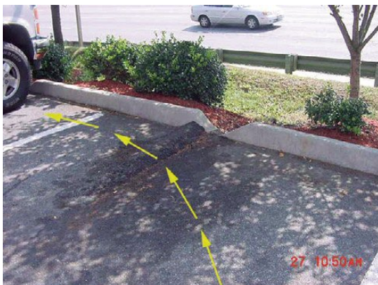
Site runoff bypasses bioretention swale.
