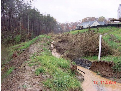
Bioretention swale clogged with sediment.
