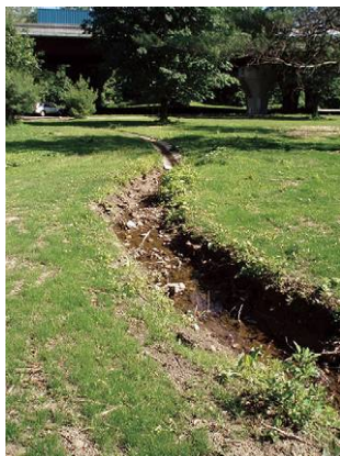
Poor Conveyance: Improperly designed conveyances become Maintenance problems in the future.
