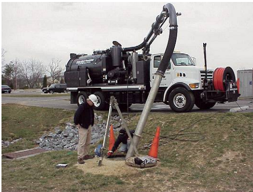
Practice Selection: Underground BMPs can be out of sight, out of mind when it comes to maintenance.
