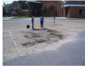
Clogged pavers and non-infiltrating infiltration bed
