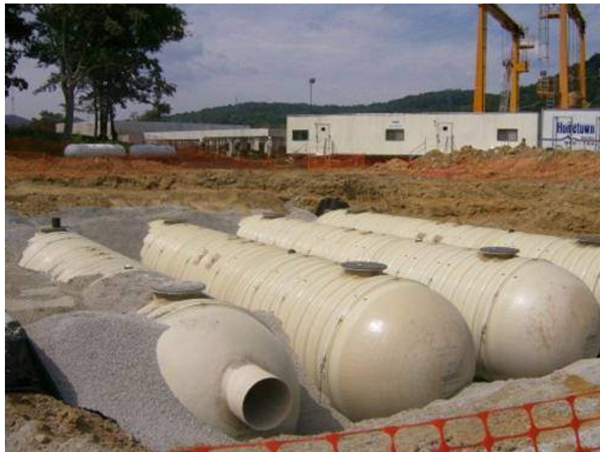
Figure 6.12. Example of Multiple Fiberglass Cisterns in Series
