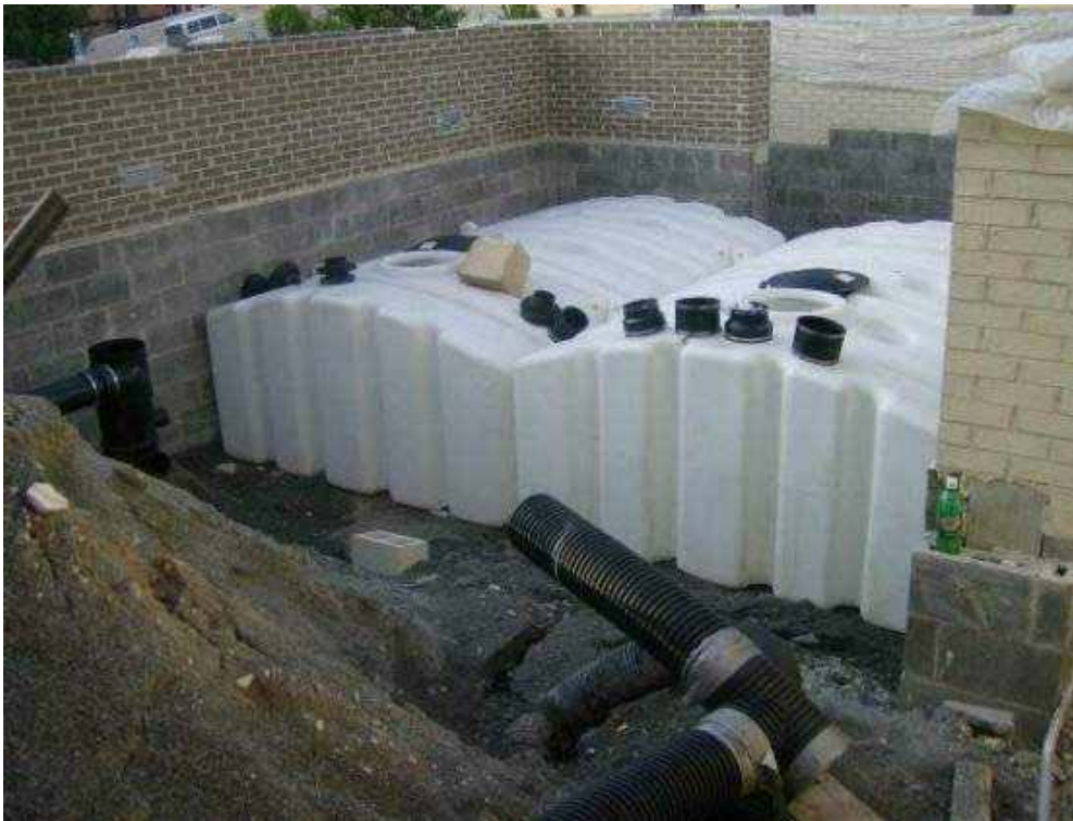
Figure 6.12. Example of two Polyethylene Cisterns
