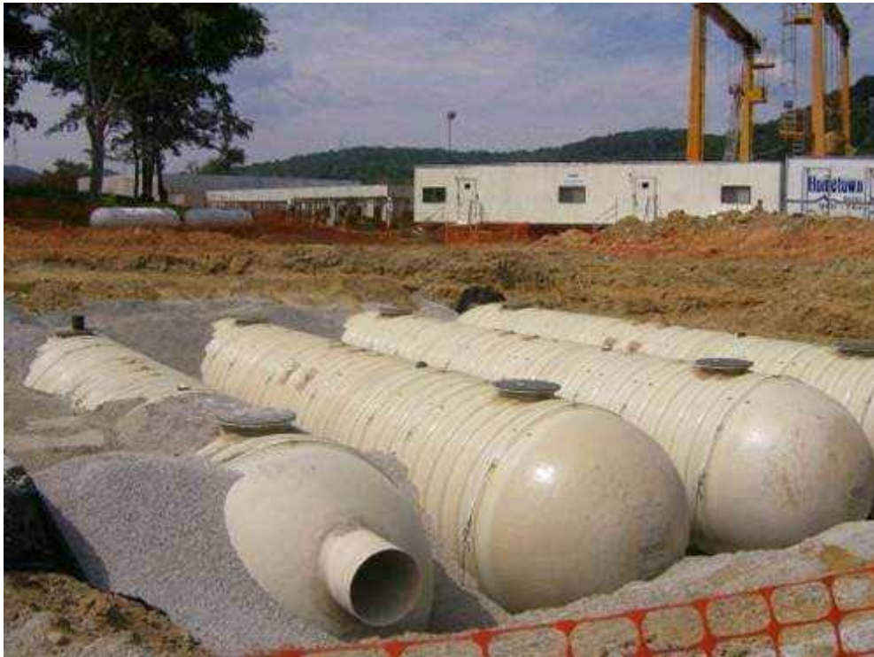
Figure 6.11. Example of Multiple Fiberglass Cisterns in Series
