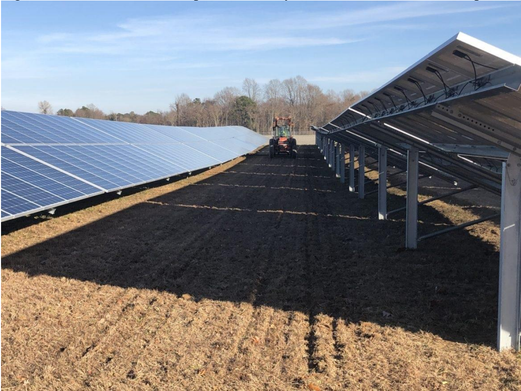
Figure 1. Pollinator Smart-Cople Elementary School Solar Panels before planting
