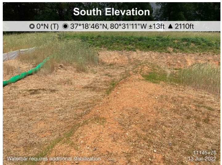
Figure 4: St 11145+67 denuded soil on waterbar requires stabilization.
