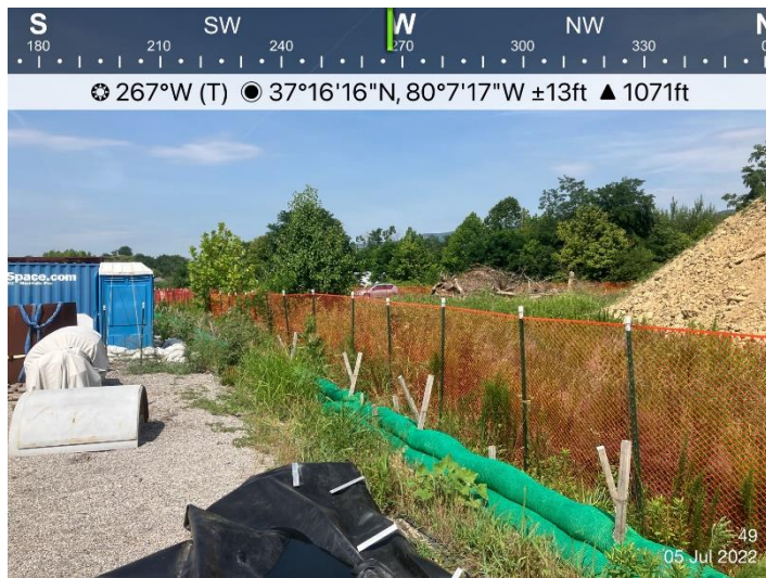
Figure 7: Laydown Yard 049 – Looking W towards entrance of LY-049. Controls are in place and functioning properly. Note offsite un-stabilized stockpile on left.
