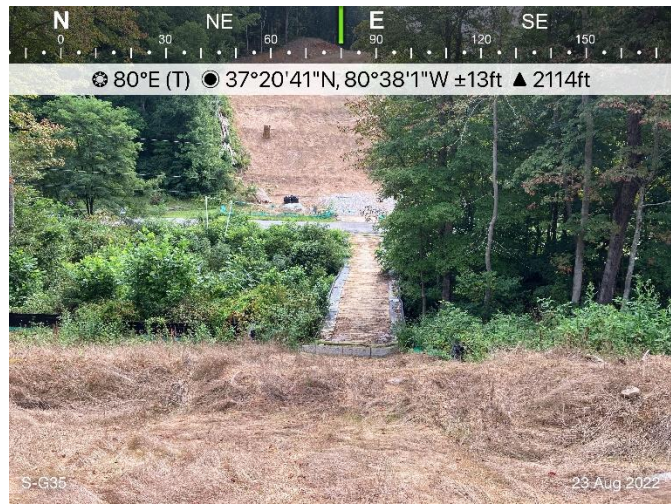
Figure 4: Designated crossing S-G35, ECD's are in place.
