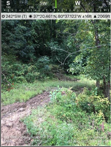
■ Figure 5: St10807+68 sediment has escaped off LOD.
