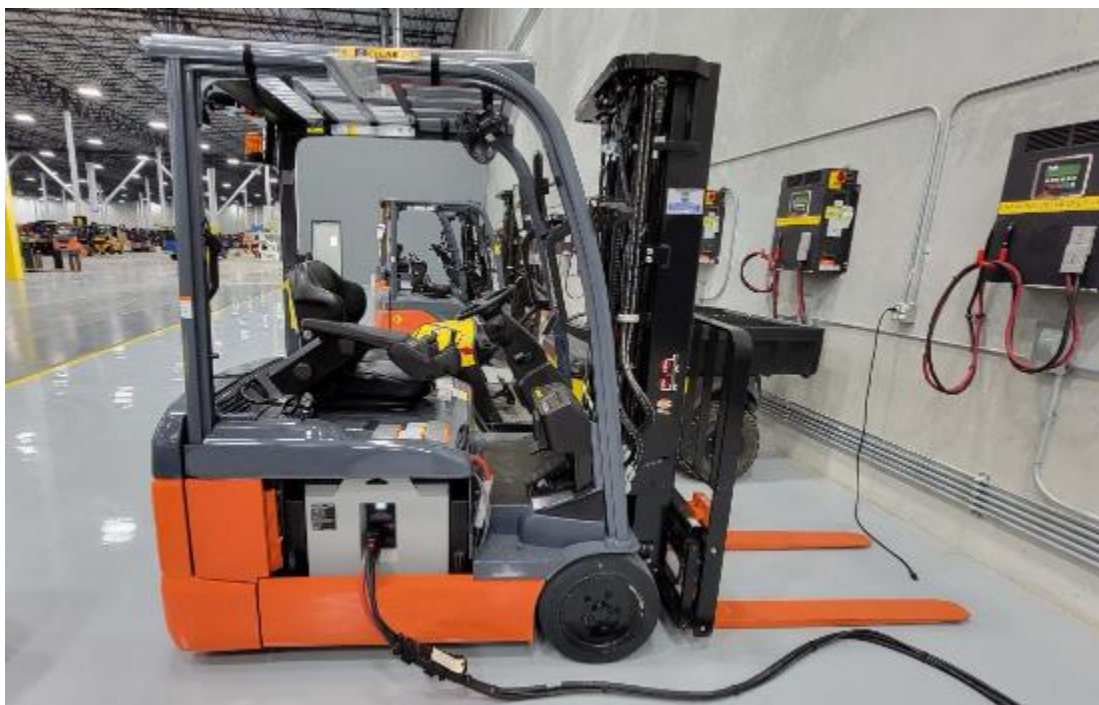
Forklift plugged in to opportunity charger.
