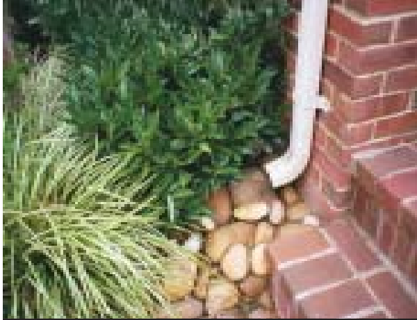
Figure 6.7: A disconnected downspout in Rivergate.
