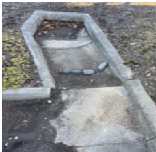
Figure 32. An environmental containment “sock” positioned in drainage ways to filter saline runoff at the VT CRC. In March, socks were collected and analyzed for mineral composition.
