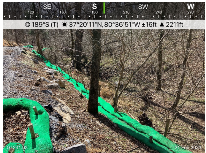
Figure 4: AR-GI 241.03 ECD's are in place.
