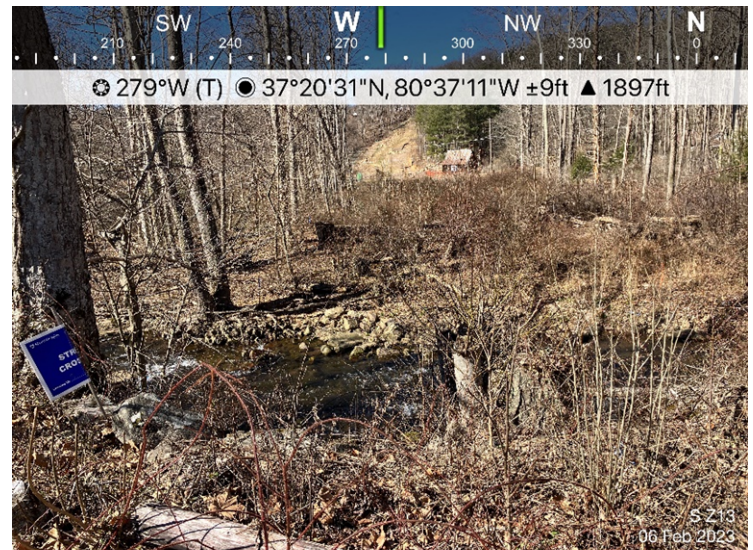
Figure 4: Designated crossing S-Z13, ECD's are in place.
