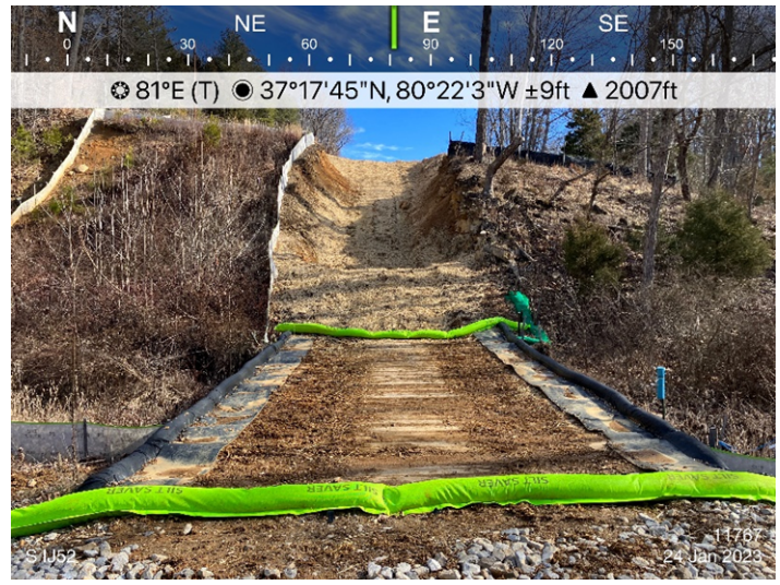
Figure 2: Designated crossing S-IJ52, ECD's are in place.
