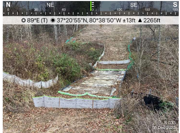
Figure 2: Designated crossing S-G33, ECD's are in place.
