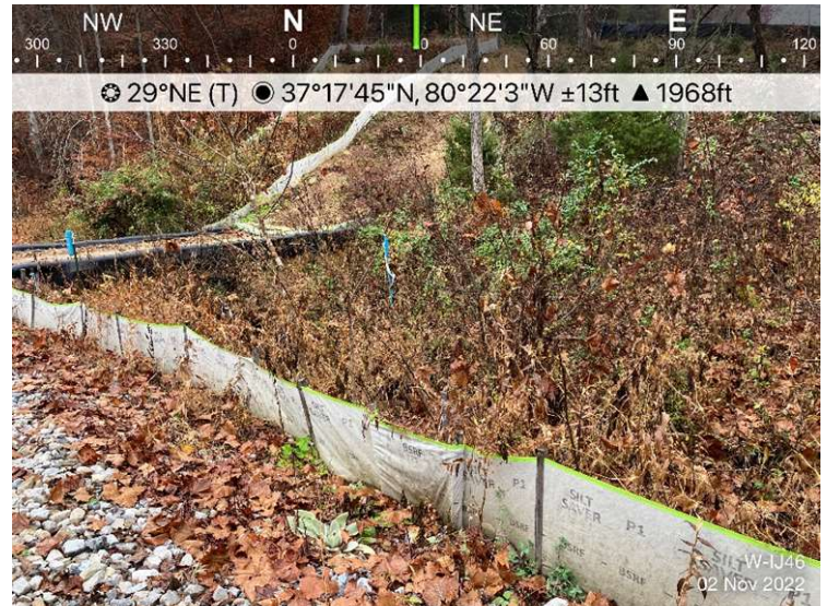
Figure 2: Designated crossing W-IJ52, ECD's are in place.
