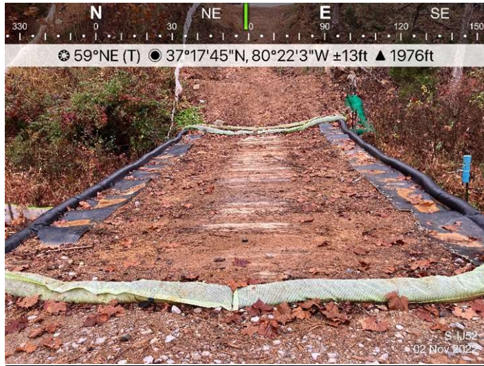
Figure 1: Designated crossing S-IJ52, ECD's are in place.
