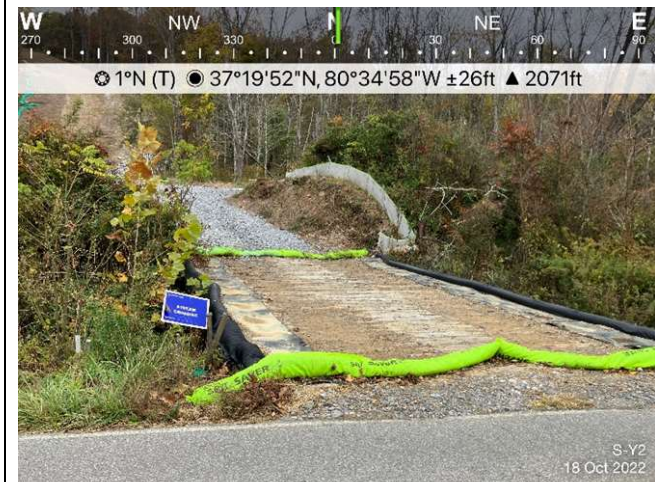
Figure 3: Designated crossing S-Y2, ECD's are in place.
