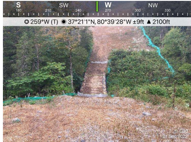
Figure 2: Designated crossing S-G30, ECD's are in place.
