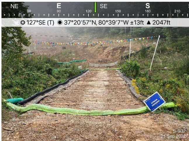
Figure 3: Designated crossing S-G32, ECD's are in place.
