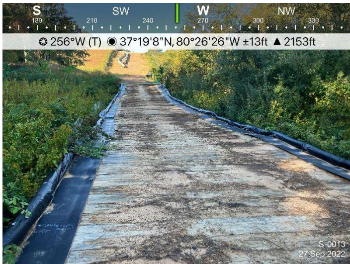
Figure 3: Designated crossing S-0013, ECD's are in place.
