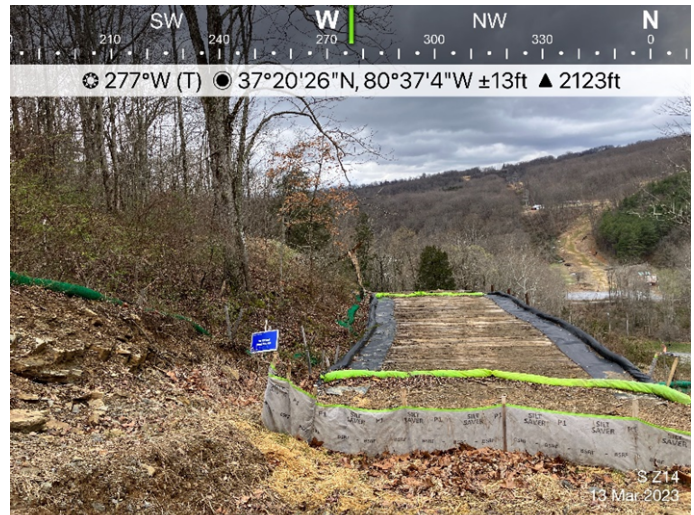
Figure 2: Designated crossing S-Z14, ECD's are in place.
