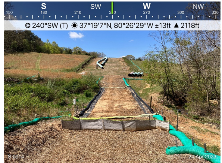
Figure 4: Designated crossing S-0014, ECD's are in place.
