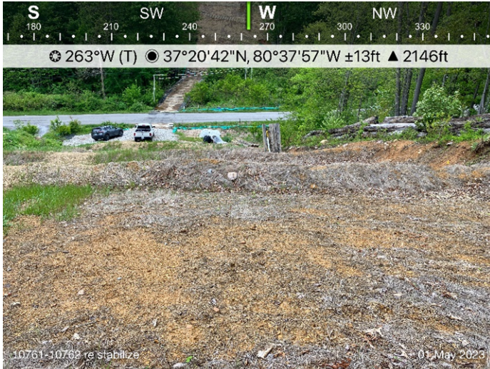
Figure 1: Sta10761-10762+50 requires additional stabilization
